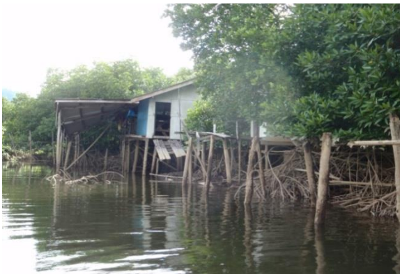
Photo. 5 Damaged Mangrove Learning Center in program (1-5) in Pang Nga province, Thailand
